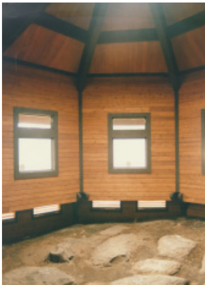
The deck (which is not shown) allows the visitors to view the petroglyphs without disturbing the rocks.
